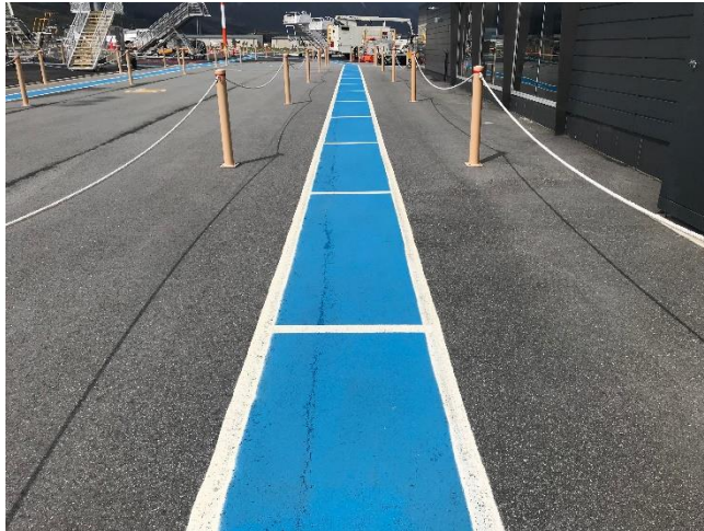
16-10 - Passenger Walkway line
